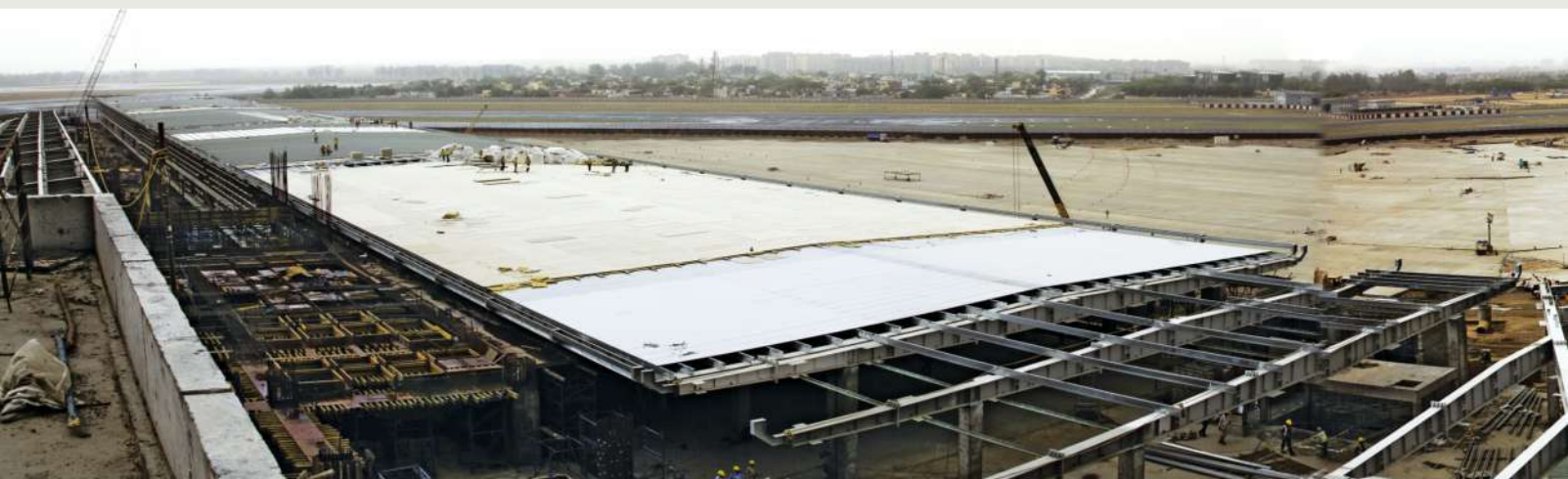
Pre-Engineered Structural Steel & Multi Layer Roofing Systems - IGI Airport Terminal 3 - Panoramic View International PIER Roof
