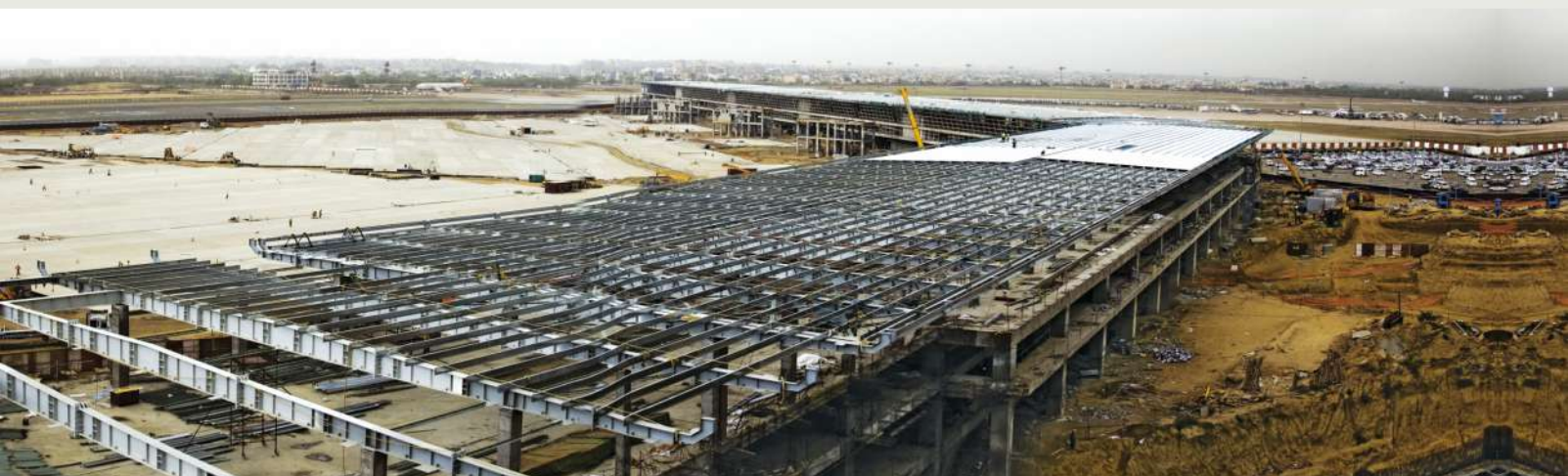
Pre-Engineered Structural Steel & Multi Layer Roofing Systems - IGI Airport Terminal 3 - Panoramic View International PIER Roof
