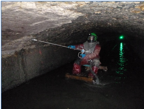
Interflow employee working on Northern Suburbs Ocean Outfall Sewer in live flow.
