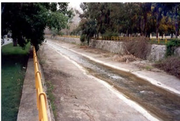
Figure 2. Nedon River (Kalamata City, Messinia, Peloponnese), a typical case of high water quality and extremely poor benthic fauna, (only 3-4 species), in a heavily modified river corridor
