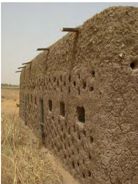
Figure 4. Reseda onion store. Built of low cost mud bricks. Windows and aeration holes are cut in the wall. Quite effective but wasteful in space.
