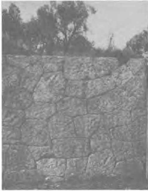
Fig. 125 - Use of polygonal blocks in Attic architecture of the 6th century B.C. - (underground tank in the Acropolis). From R. Martin, Manuel d'Arch. Grecque Picard Paris 1965 - PI XXXVIII,3.
