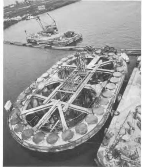
Fig. 4 Steel pipe pile caisson under construction (courtesy of Kawasaki Steel Works Co.)
