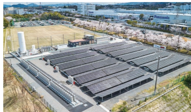
Panasonic Corporation Kusatsu Plant (power supplied by pure hydrogen fuel cells and solar panels)
