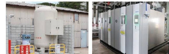
LPG supply facility
