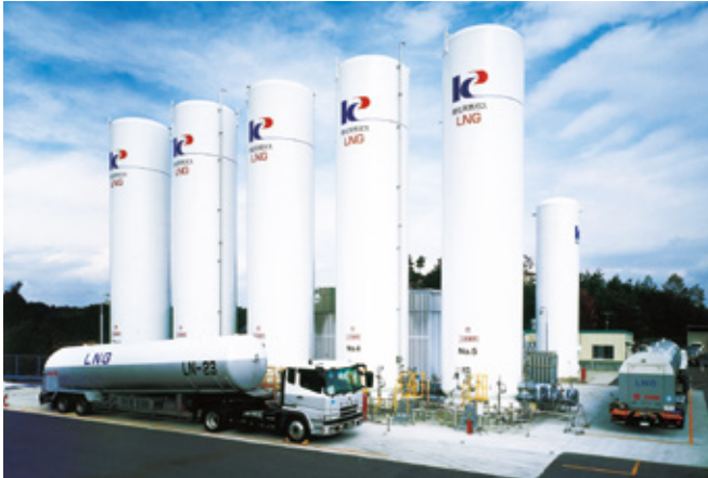
An LNG Satellite Facility (operated by Koga Energy Co., Ltd.)
