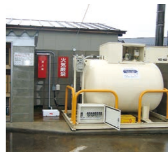
Disaster-ready LPG bulk storage tank
