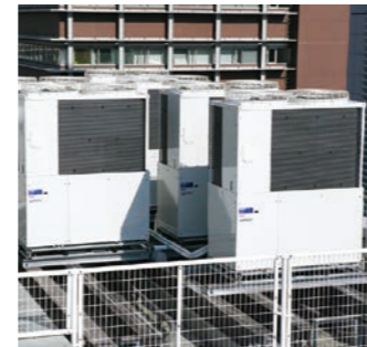
Gas heat pump (GHP) air conditioners
