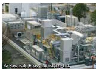
Photo of the Kobe Smart Community Hydrogen Power Generation Project (Port Island), a NEDO subsidized project (conducted by Obayashi Corporation and Kawasaki Heavy Industries, Ltd.)
