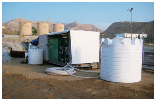
Setup of the water treatment unit
