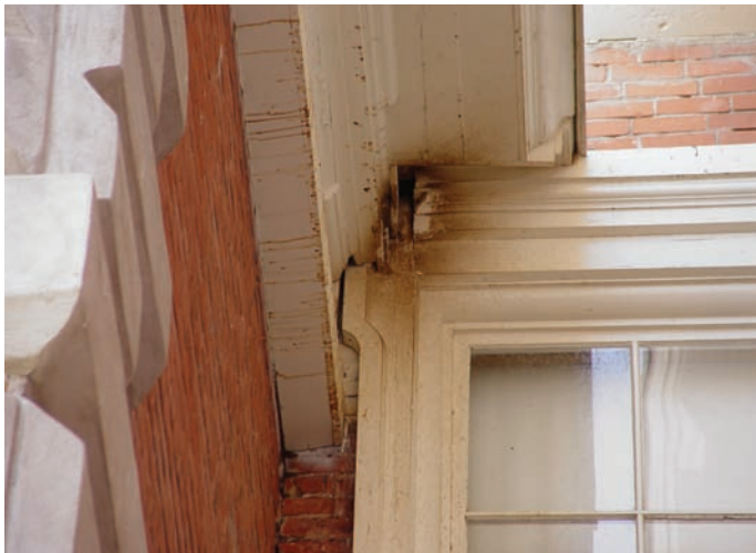
A halo-like rub mark around an entrance hole reveals a bat roost; guano accumulates below a frequented roosting site; a white urine stain in a corner beneath a roost.
