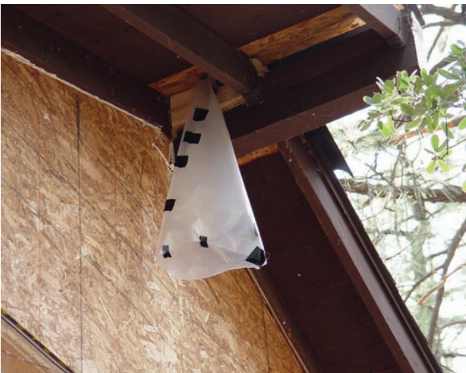
Open-bottom screens and self-made sleeves are effective and affordable tools that prevent re-entry to the roost, while also allowing interior bats to exit.
