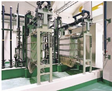
High-load membrane night soil treatment facility
