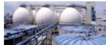
Sewages sludge methane fermentation facility
