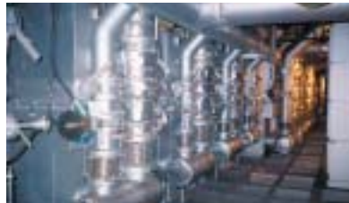
Regenerative burner heating system
