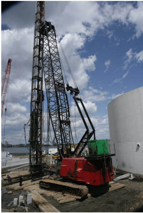
A crane was brought in to drive 192 piles to create the supporting columns for the building's foundation.
