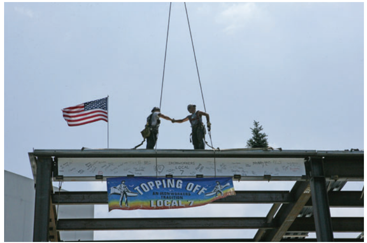
Iron workers top off the steel skeleton of the new addition on July 16, 2010.
