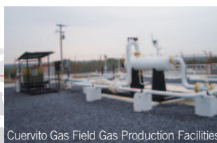
Cuervito Gas Field Gas Production Facilities
