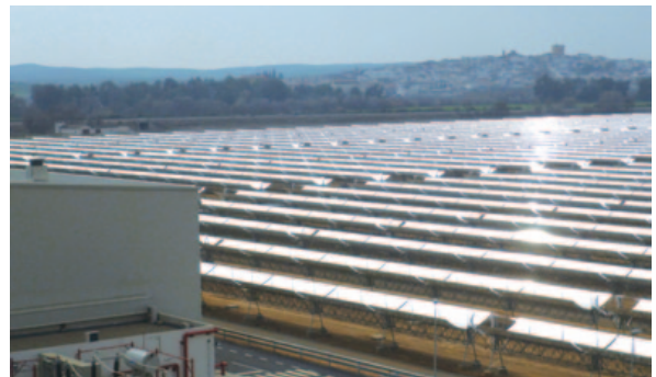
Concentrating solar power facility (Spain)
