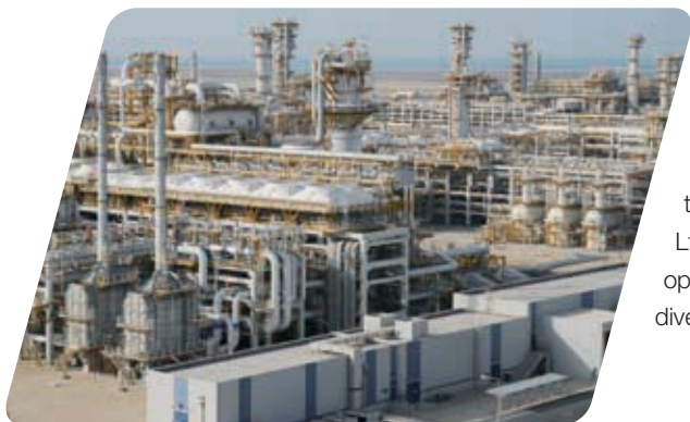
Natural gas processing plant for Dolphin Energy Limited, Qatar
