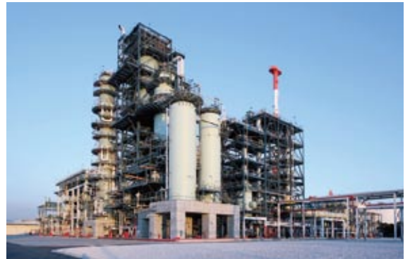
Petroleum refining-related plant for Fuji Oil Company, Japan
