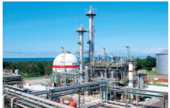
A DME manufacturing plant for Fuel DME Production Co., Ltd., Japan
