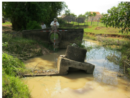
Damaged culvert on canal
