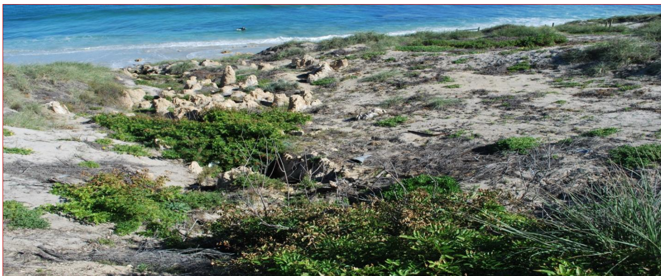
Figure 6: Signs of erosion in vicinity of drain line and presence of Japanese Pepper Trees
