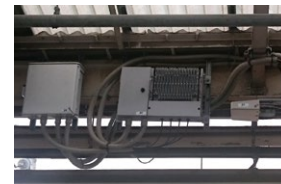
Improvement of a WiMAX base station
