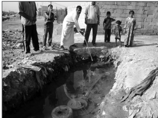
Figure 24. U.S. and Iraqi forces ongoing repair of major sewer and water point breaks in Sha'ab/Ur districts of Baghdad
