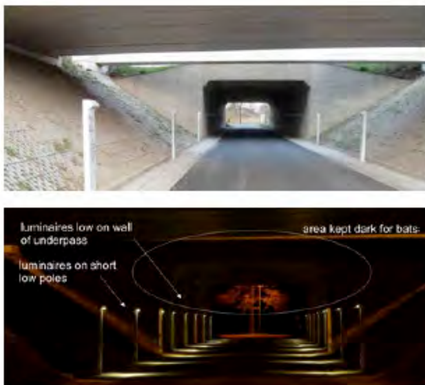
Figure 50: Installation of luminaires on short poles to reduce artificial light at night on a commuting route for bats through an underpass in the Netherlands (the same place in daylight and at night). Source: Voigt et al. (2018); photograph by F. Brekelmans
