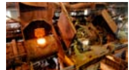
Anode furnace, Tamano Smelter
