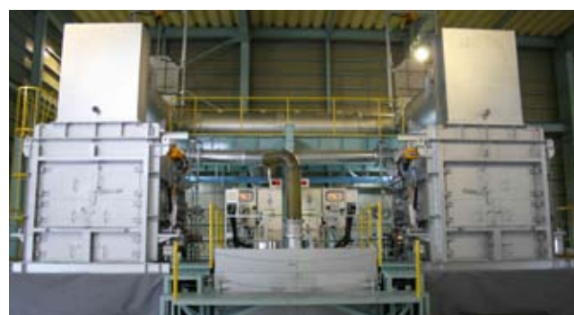
New stationary furnace
