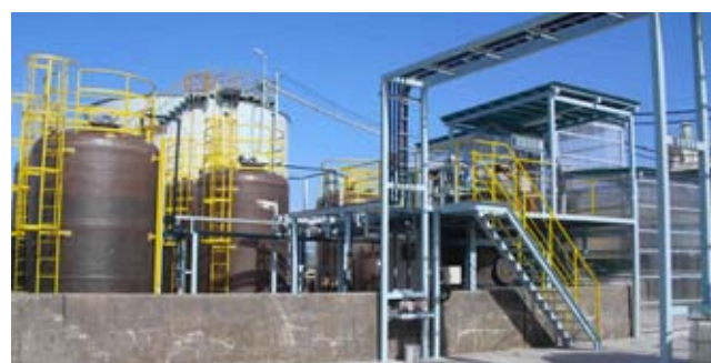
Indium and cobalt recovery plant
