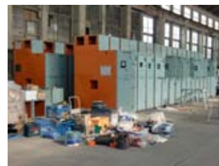
Transformation equipment delivered from the Negishi Refinery, JX Nippon Oil & Energy ( feeder board )
