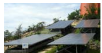
Panels for photovoltaic power generation at the Hibi Kyodo Smelter
