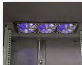
3 x Super-Silent fans in roof area
