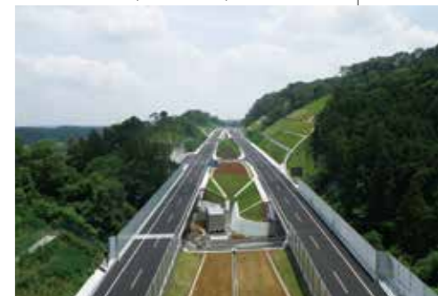
Roadwork between the Sagami-hara-ai-kawa Interchange and Sagami-hara Interchange on the Ken-O Expressway.
