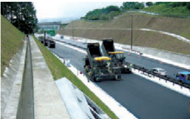
Road pavement work on the Izu Jukan Tokura Road (Constructed by Kajima Road Co., Ltd.)
