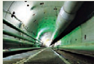
Gas pipeline inside the tunnel
