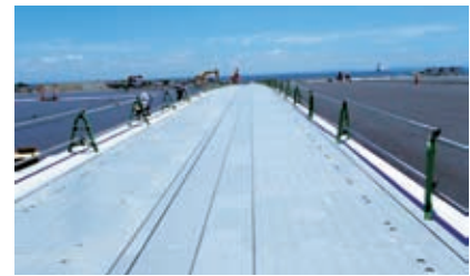
“Roller-shutter type” expansion joint (linking the reclaimed island and piled-elevated platform of the runway) during construction
