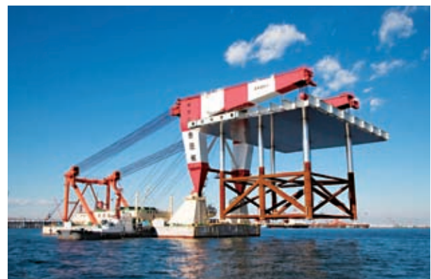
Piled-elevated platform during construction. The runway was created after connecting the component to a steel jacket.
