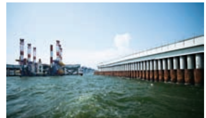
Wave-absorbing seawall during construction. 229 concrete pillars were installed for the seawall (428 m) on the reclaimed island side.
