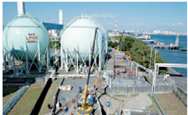
Construction work to prevent coastal erosion at the LNG Terminal (Constructed by Chemical Grouting Co., Ltd.)
