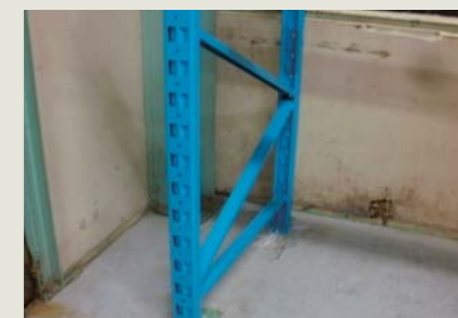
Some racks had no anchor bolts and were prone to tipping over. We checked and upgraded all racks, fixing them with anchor bolts
