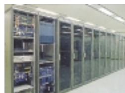
Interior of colocation room (KDDI Building, Shinjuku)
