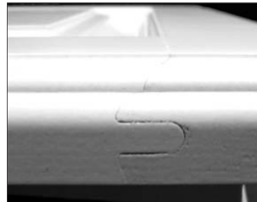
Example of end joint separation
