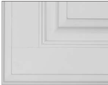
Example of front joint separation
