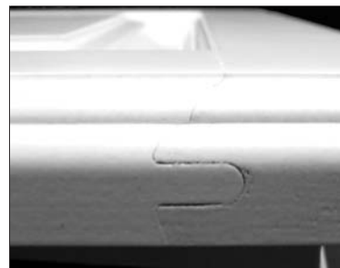
Example of end joint separation
