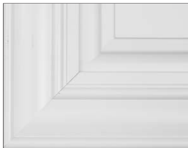
Example of front joint separation
