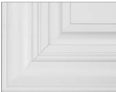
Example of front joint separation
