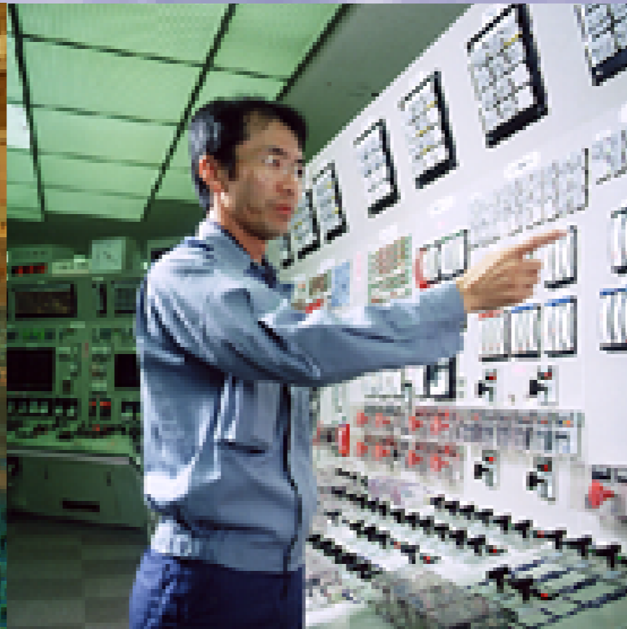
Central Control Room (Takahama Nuclear Plant)
