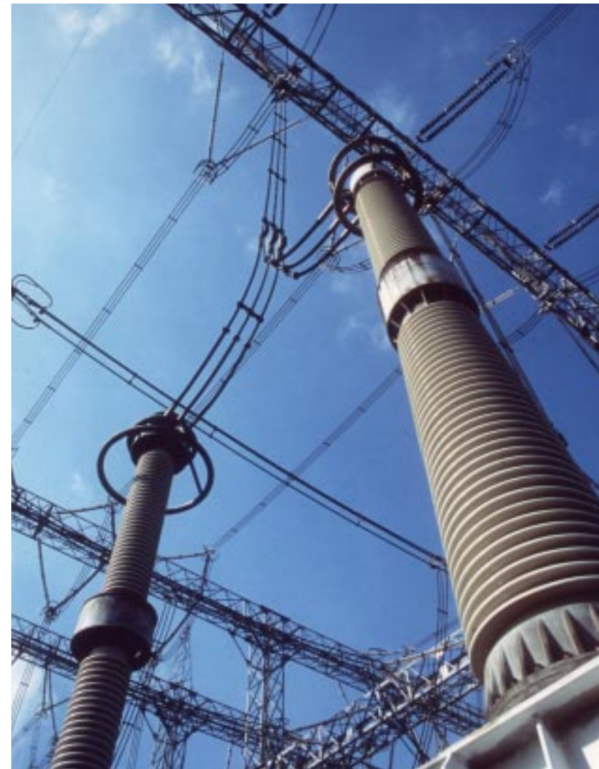
(from top) Transmission network map Shin-Ikoma Substation
