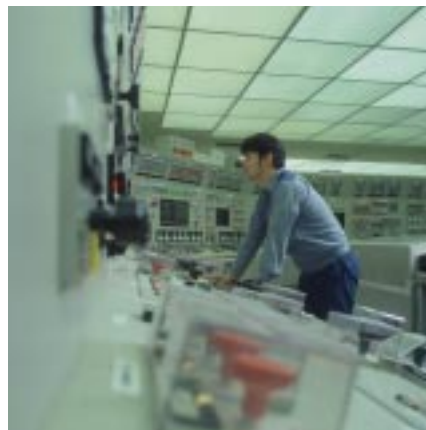
Central Control Room (Takahama Nuclear Plant)
