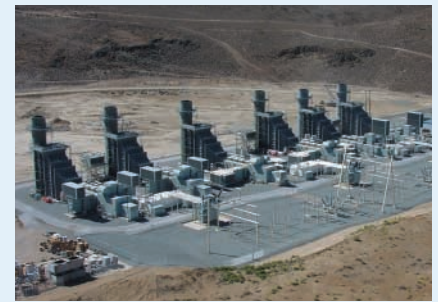
Gas turbine with a second reused on life
