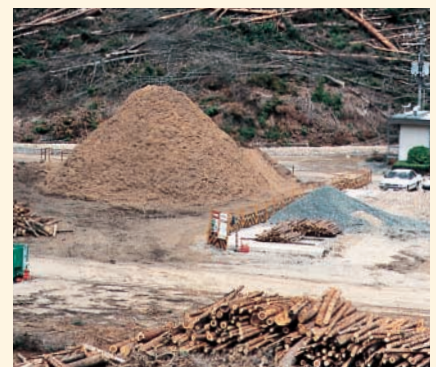
Excavated soil and fallen trees from ground work being reused for construction
