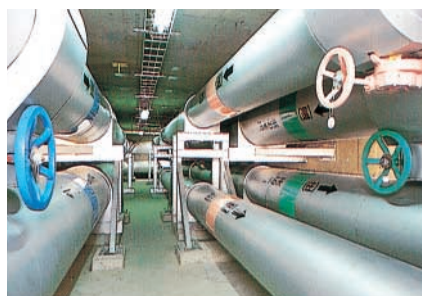
Utility tunnel and pipes
