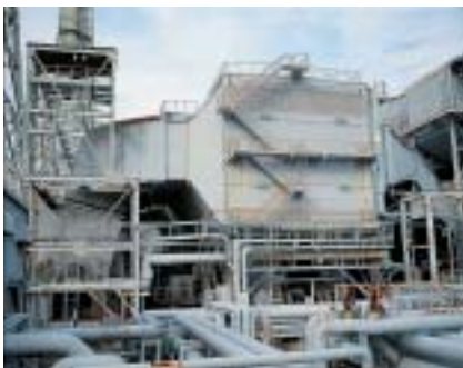
Electric dust catcher at the Kainan Power Station
