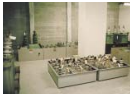
PCB waste storage facility
