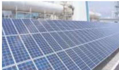
Solar panels on a roof at the Nanko Power Station
