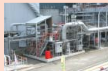
Reused boiler at Aioi Power Station
