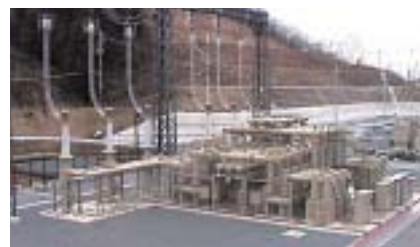
GIS at the Nose Substation
