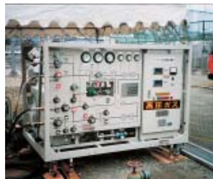
One of 26 SF 6 gas recovery systems installed at Kansai Electric facilities
