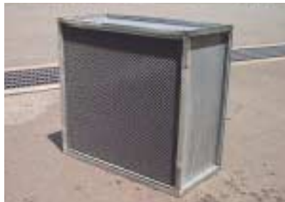
Intake filter (Himeji No. 1 Power Station)
