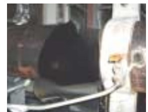
Site of condensate piping rupture
