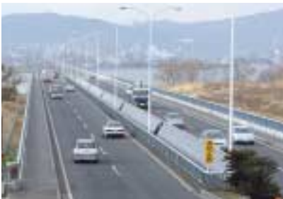
Solar power generation equipment (Shiga Prefecture, Ohmi Bridge)
