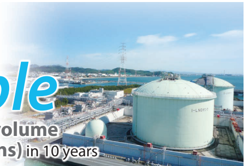
LNG tanks on the grounds of the Himeji No. 2 Power Station
