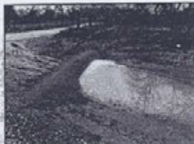
Vegetated compost filter berm; note clear water on downstream side of berm. Source: TCEQ
