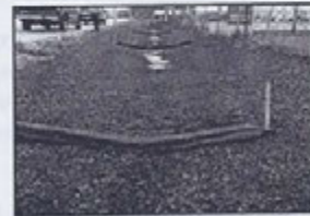
Installation of filter socks in a road ditch; socks will be staked through the center. Source: Filtrix International, LLC
