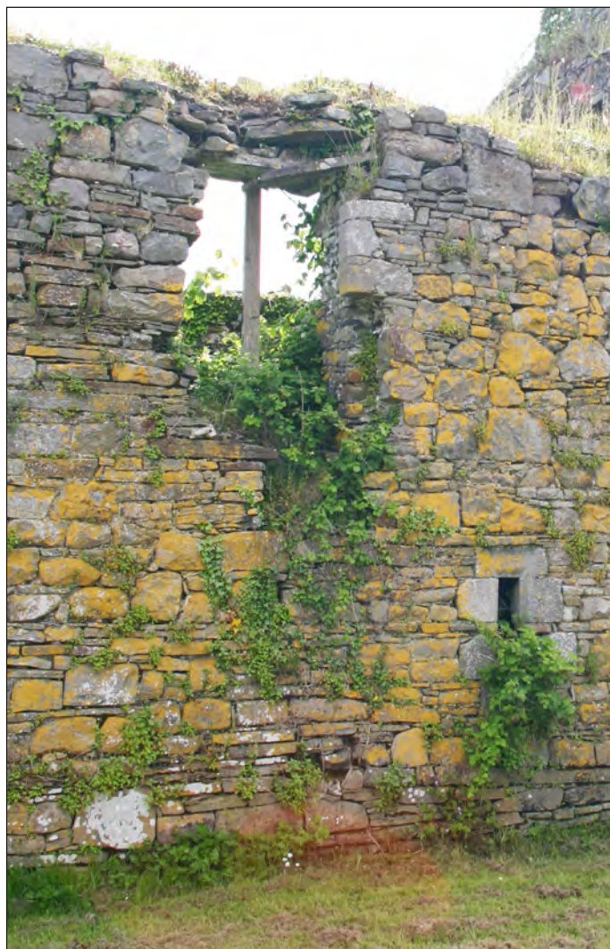
Plate 31: Close up view of upper level partially collapsed and ragged window at western limits of north elevation. Note temporary and ineffectual prop
