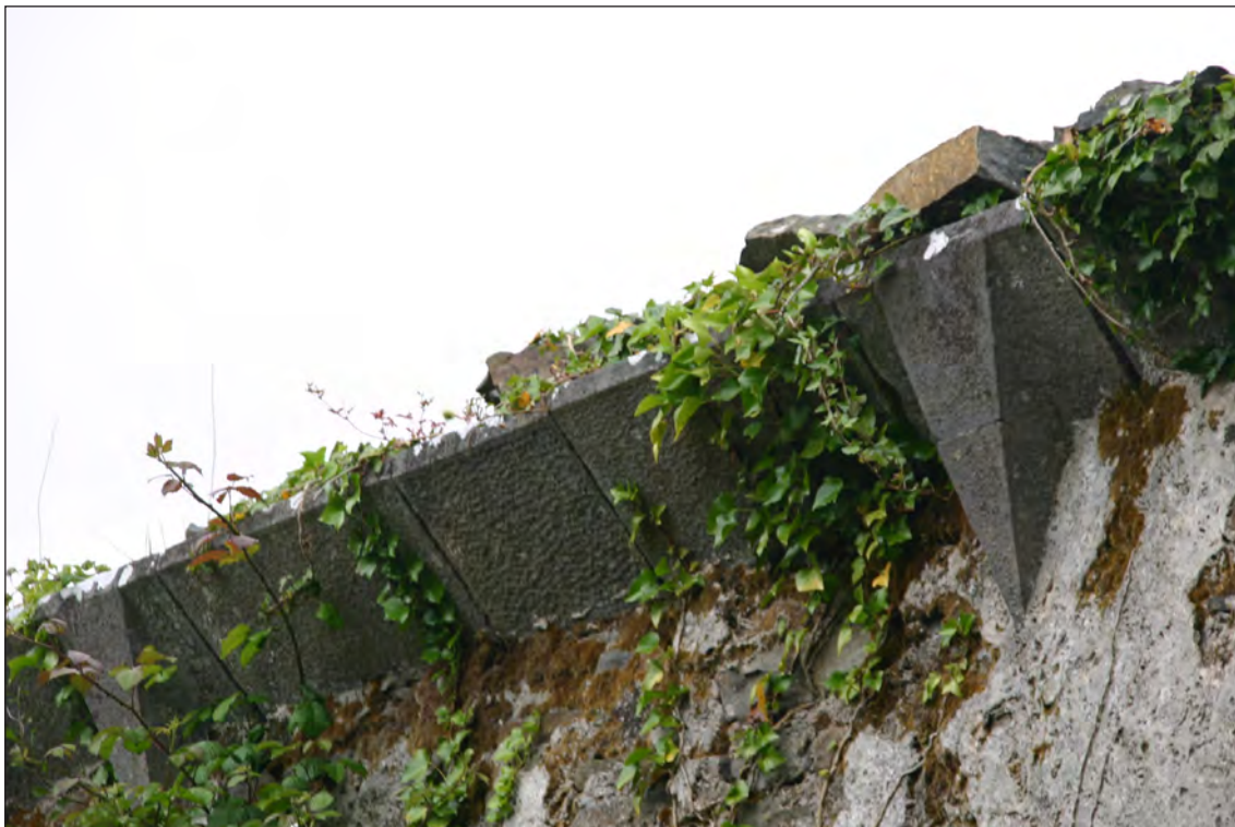
Plate 27: View of the dressed limestone, corbel course including featured larger pointed corbels on interior of Aghavallen Church. This very fine architectural feature is identical to Carrigafoyle and Kilnaughtin churches
