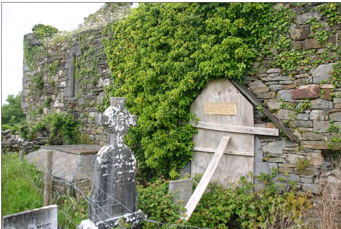
Plate 25: View of the boarded up doorway on the south elevation of Aghavallen Church. Note the overgrown nature of area including wall and ground compounded by the insertion of a temporary and ineffective post and wire fence
