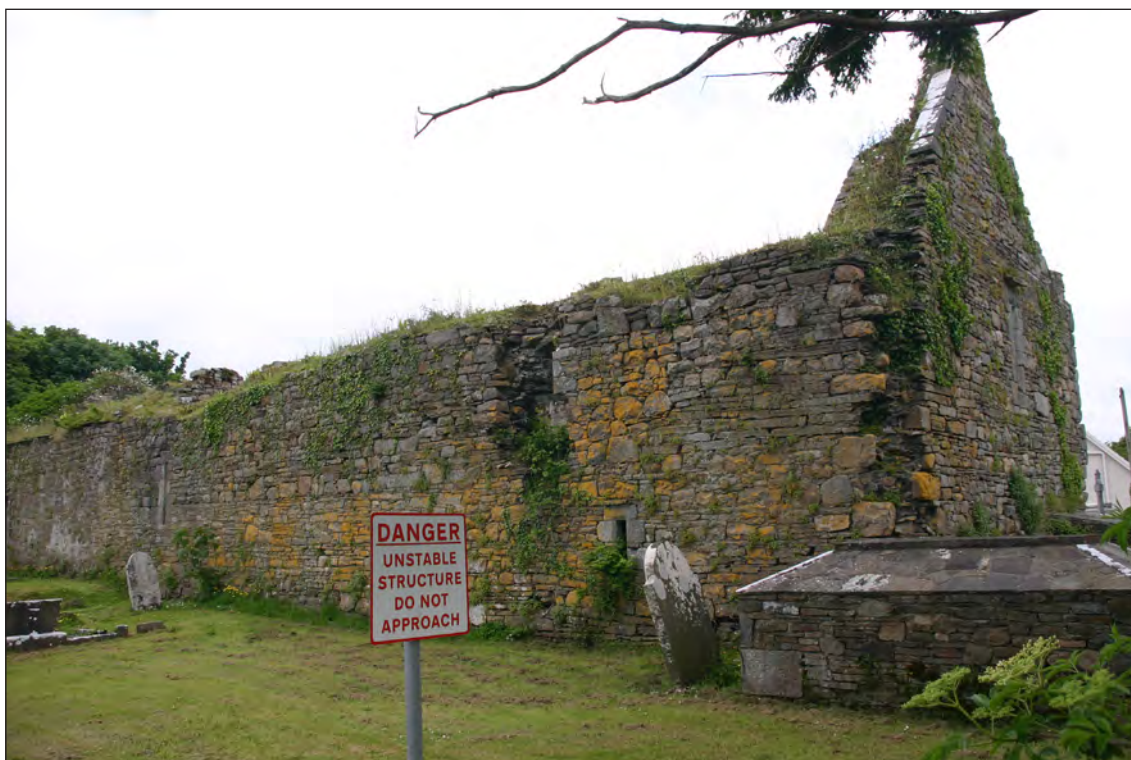
Plate 26: View of north elevation at west end of Aghavallen Church. Note ragged and dangerous upper window, robbed out quoins and DANGER sign
