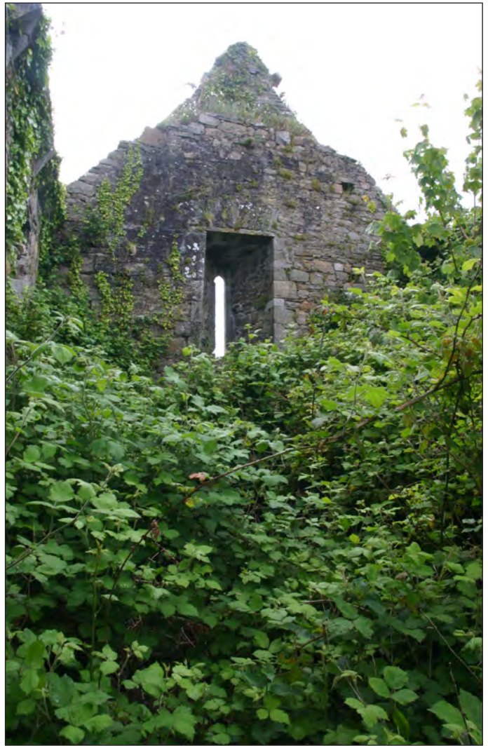
Plate 9: View of completely overgrown western limits of interior of Aghavallen Church. Note upper level window and beam slot
