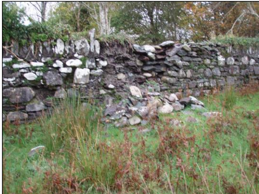
Pl. 1. Collapse of wall on S side of graveyard
