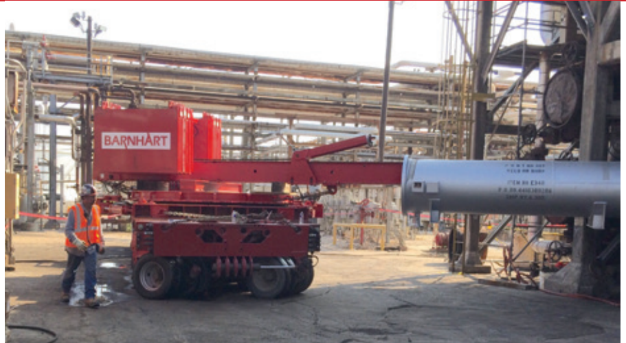
Barnhart's solution involved a custom MOCCS arrangement with 30 kips of counterweight setting atop and secured to a 750-ton hydraulic turntable setting atop and secured to six lines of Goldhofer PSTe. Barnhart named the solution 'The M3A1.'
