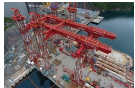
Fagioli assembled and installed modules into a topside unit on a customized pier.
