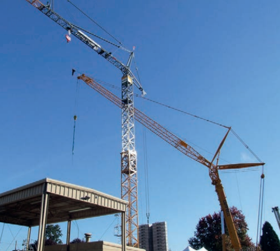
Morrow Equipment demonstrated a Liebherr 81K.1 fast-erecting crane. This was the first time that a tower crane was part of the Lift and Move USA program.
