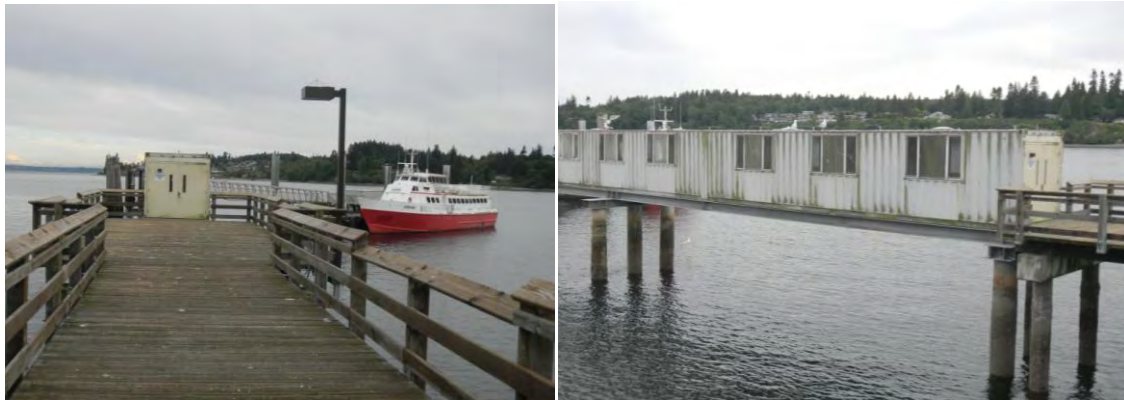
Figure 5-4: Existing Kingston POF Facilities (Wooden elevated walkway pictured left and covered walkway shipping container pictured right).
