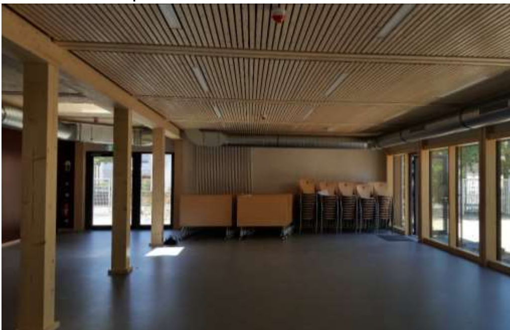
Cafeteria area with ventilation ducts
