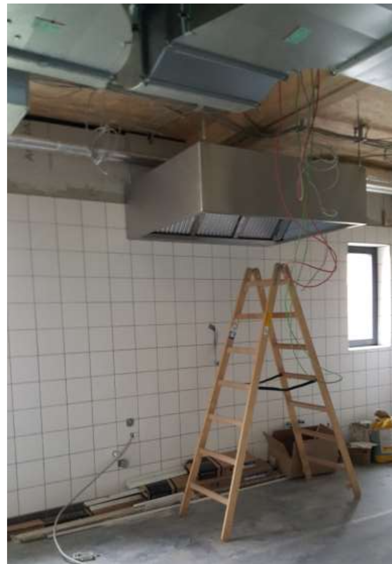
Hood above washing mashine – contrast between wooden construction and kitchen
