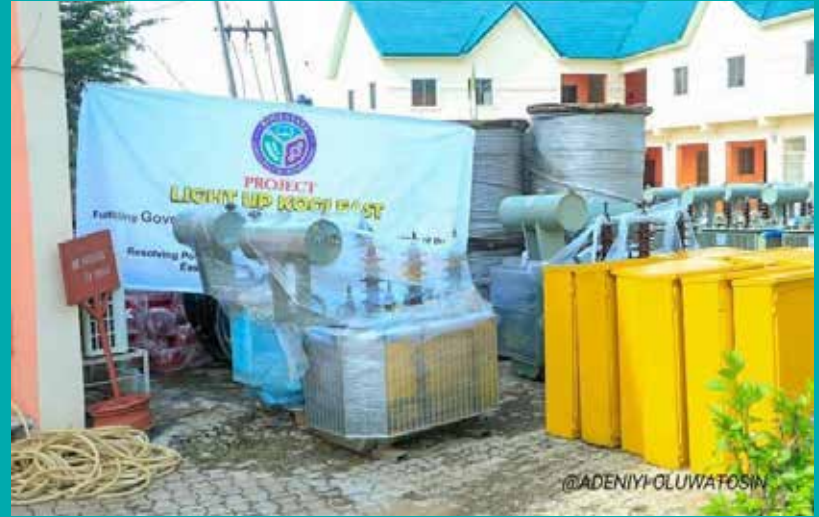
Project Light Up Kogi East Electrification supplies
