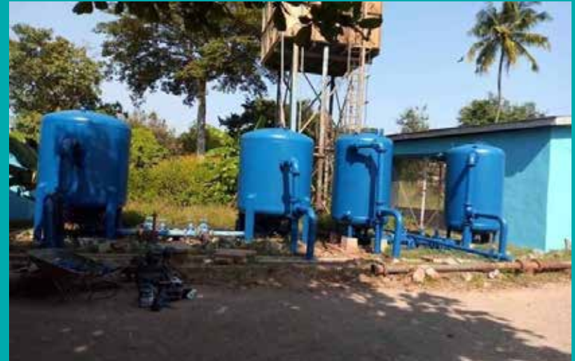
Okene Mega Water works
