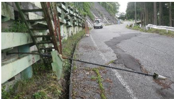
Photo 1. Damage due to anchor rupture
