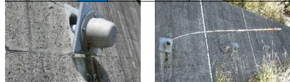
(a) Protruding anchor head and PC steel stranded wire
