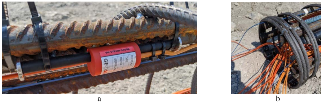
Fig. 3 Vibrating wire strain gauge linked to a rebar (a) and cables exiting the top of the steel cages (b)
