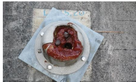
Photo 7. Breakage of anchor head by anchor rupture
