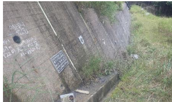
Photo 4. Condition of the slope after anchor rupture
