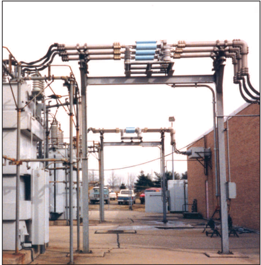
▲ 5.5kV, 3000A CLiPs protecting the utility from a small cogeneration plant.
