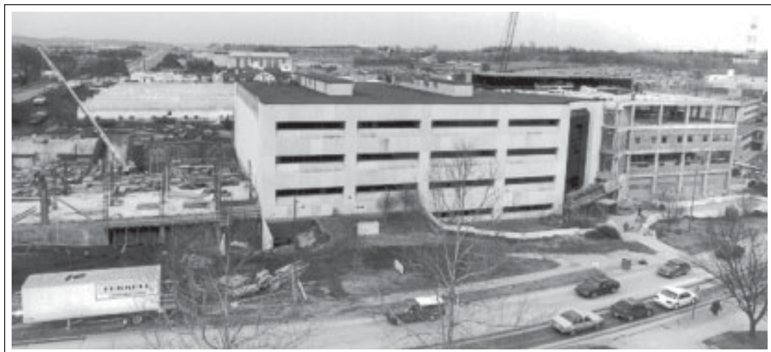
This new addition to Throckmorton Hall will provide additional space for research in plant science by several departments.
