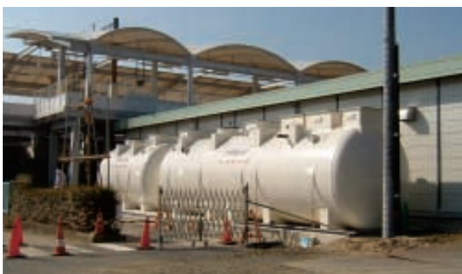
The Wastewater treatment tank with advanced membrane process installed at the Banpaku-yakusa station
