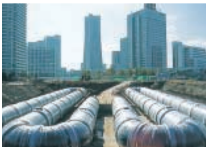
Water storage tanks using ductile iron pipes
