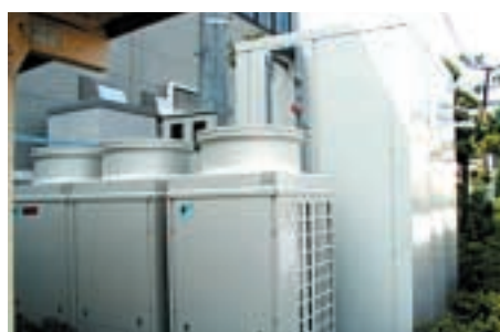
Thermal storage tank for the Eco Ice System
