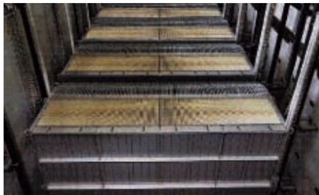
Sewage treatment equipment in the Fukusaki Water Purification Center, Fukusaki-cho, Hyogo Submerged membranes units installed in reaction chambers
